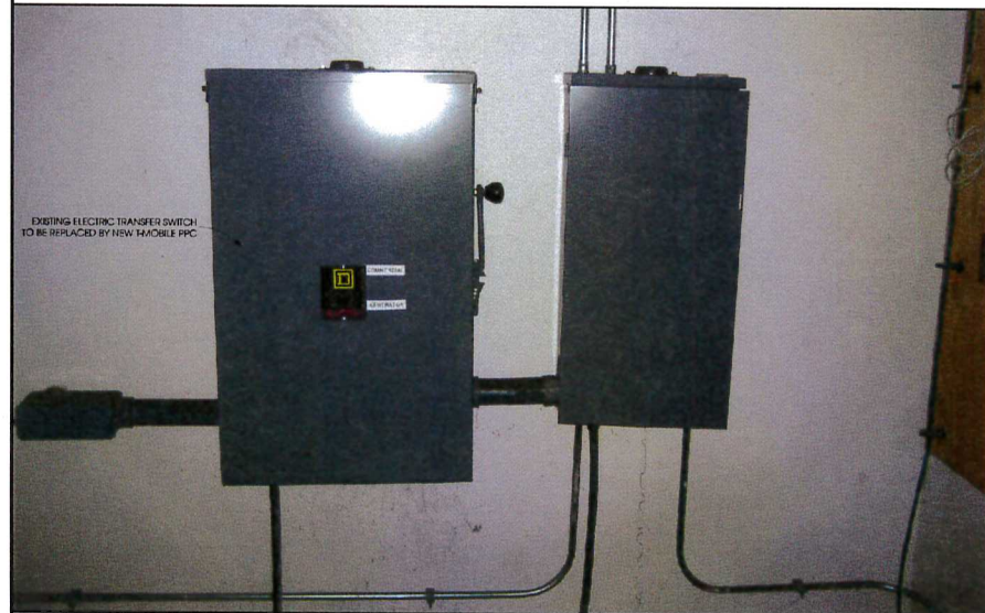
EXISTING ELECTRIC (INSIDE SHELTER)
