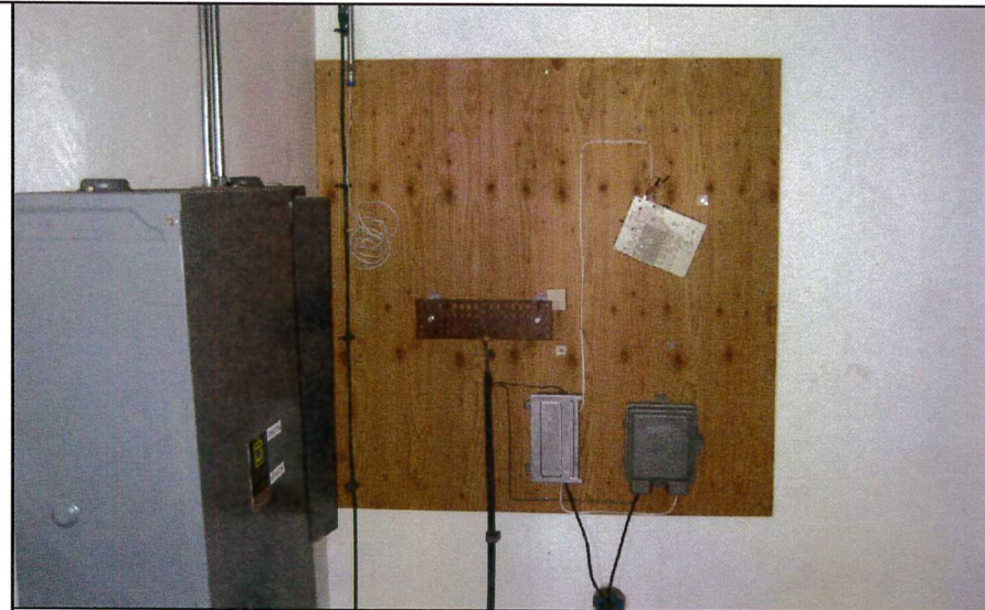
EXISTING TELCO BOARD (INSIDE SHELTER)
