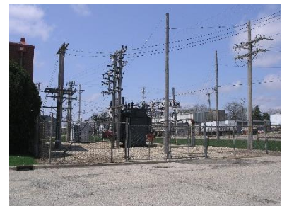
Electric substation in the City of Elkhorn
