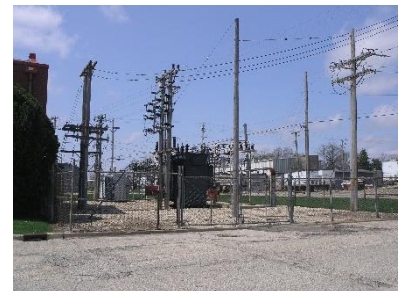
Electric substation in the City of Elkhorn
